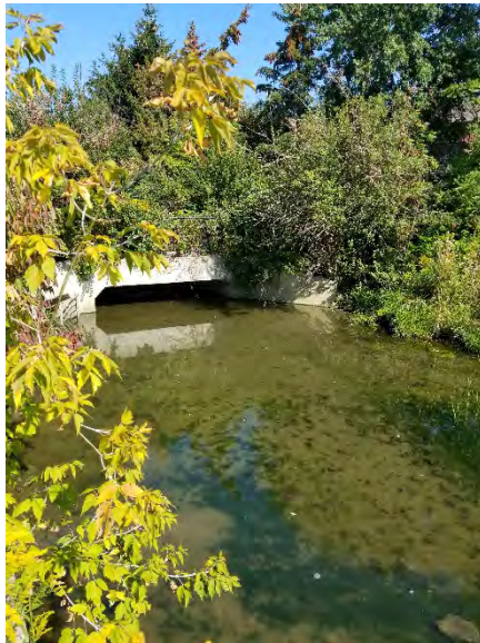
Photo 6 – A view of the southern branch of Salt Creek and the road culvert located on the east side of the Site.
