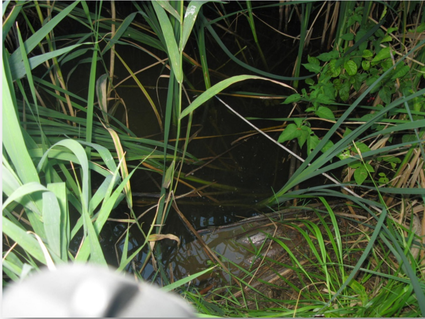
Photo 13: Culvert C6 south end – 100% submerged
